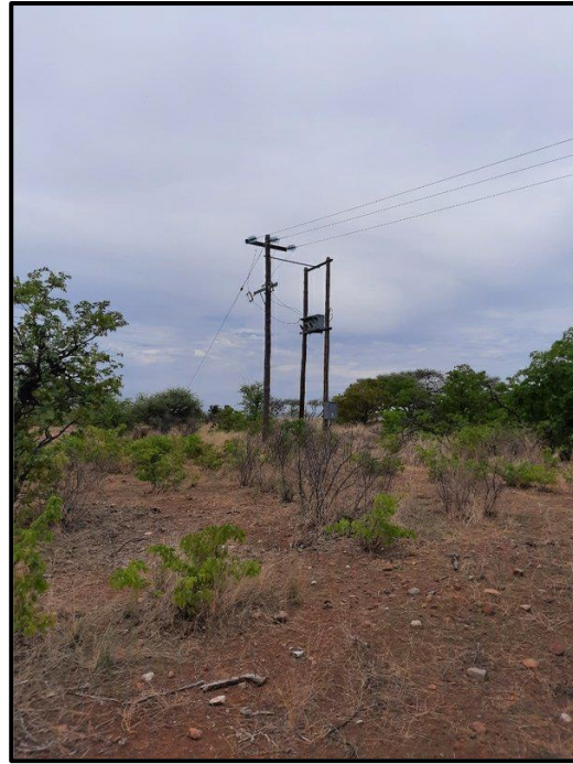
Figure 7.2. Existing powerline viewed from Option 2.
