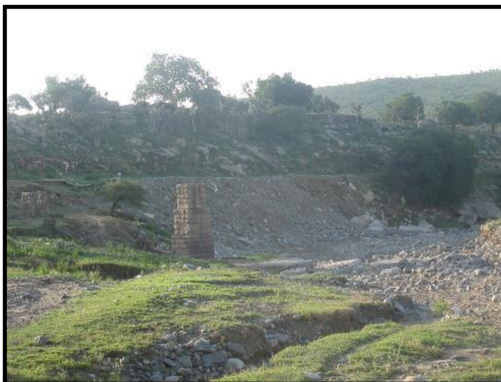
Figure 9. Photograph of old and damaged Siphon. It is situated in a dry stream bed that feeds into the Thukela River.
