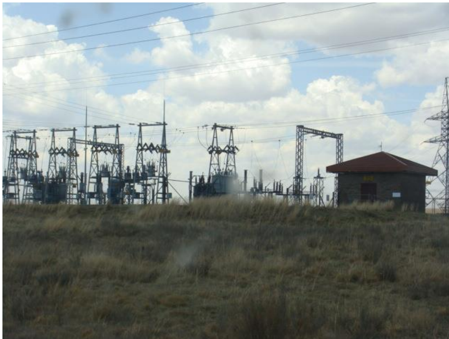
Figure 14 The Warden Rural Substation.
