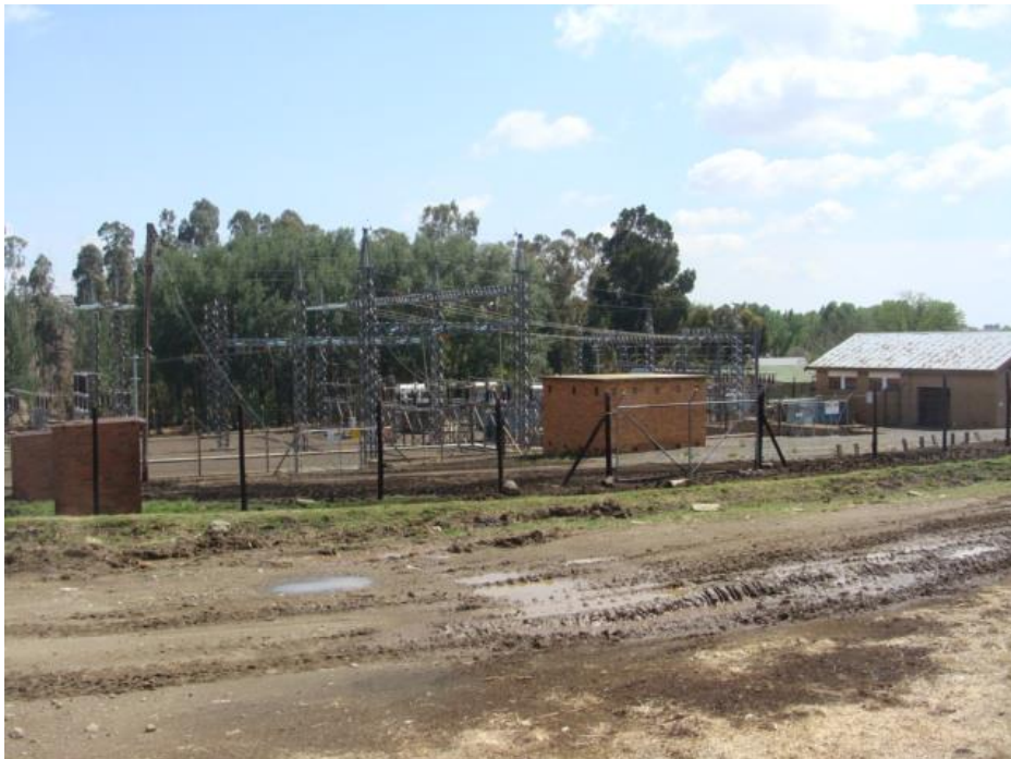
Figure 6 The Vrede Substation.
