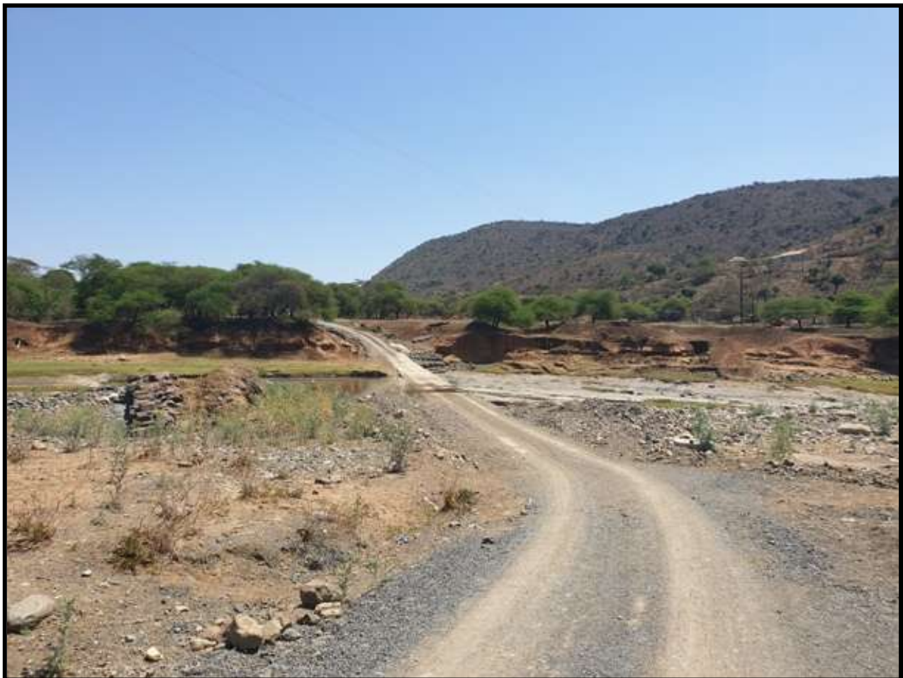
FIG. 8: EXISTING CAUSEWAY AT BLOUWKRANTS RIVER
