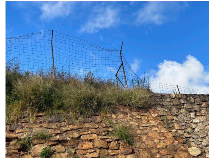
Figure 19: Damaged wire fence
