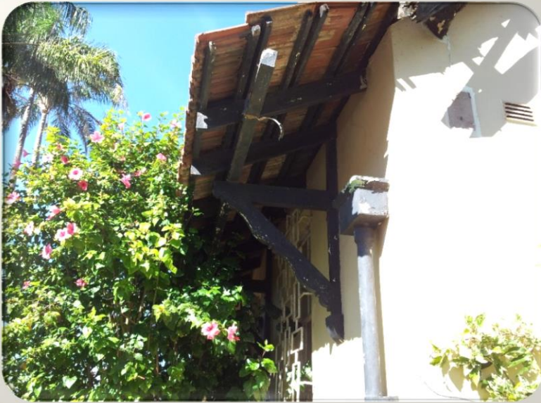
Photo showing missing bargeboard
