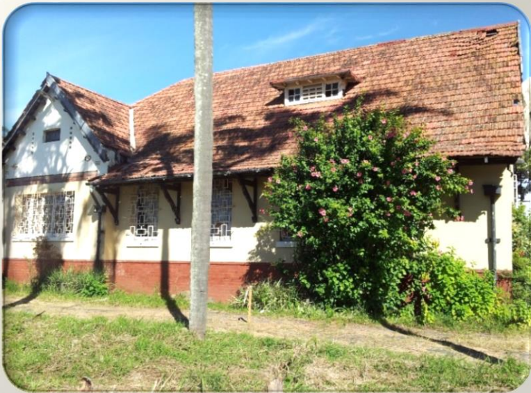
Photo of existing roof in poor condition
