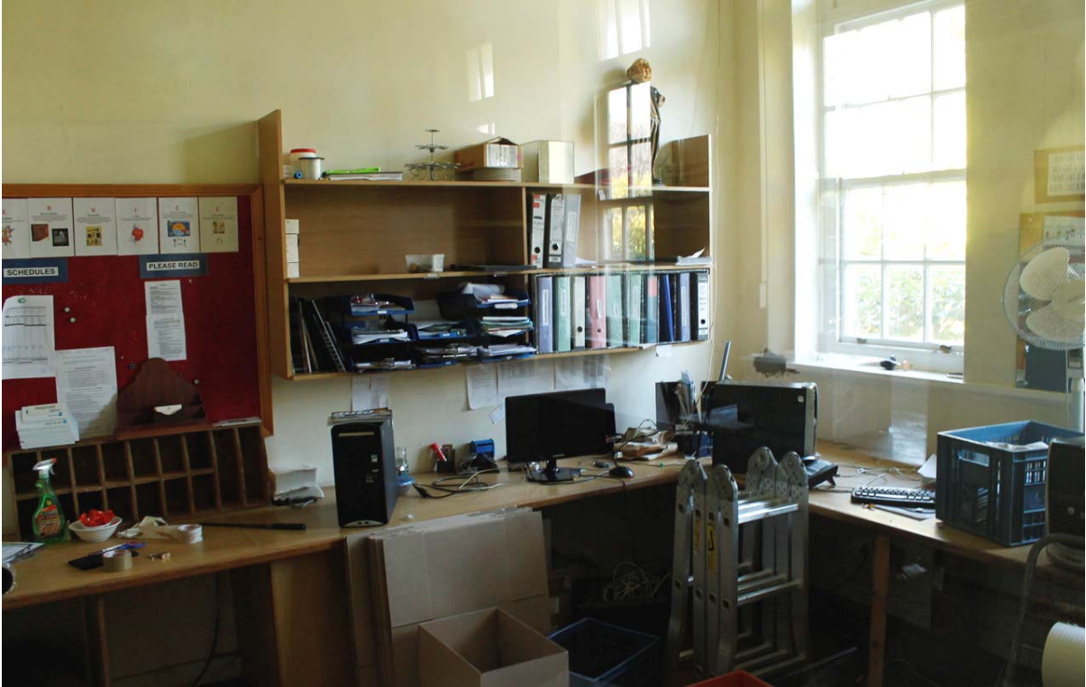
Figure 15: An existing office, located between the toilets and the kitchen. This space will be opened up and incorporated into the open-plan food hall. The outside windows will remain unchanged.
