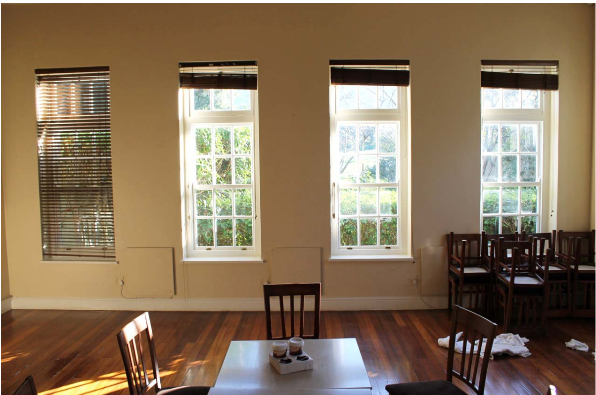
Figure 16: The dining room in the western wing. The central two windows will be replaced by double-opening French doors, centred between the remaining windows and with the same height as the windows.
