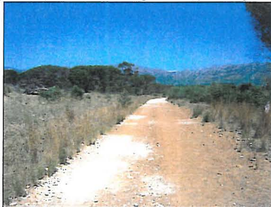
VIEW B: Section of access road to the subject property, parallel to N2
