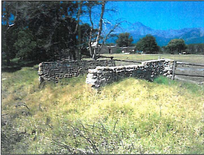
VIEW F: Stone bridge structure to be retained/ location where former historic pathway intersected with non-perennial watercourse
