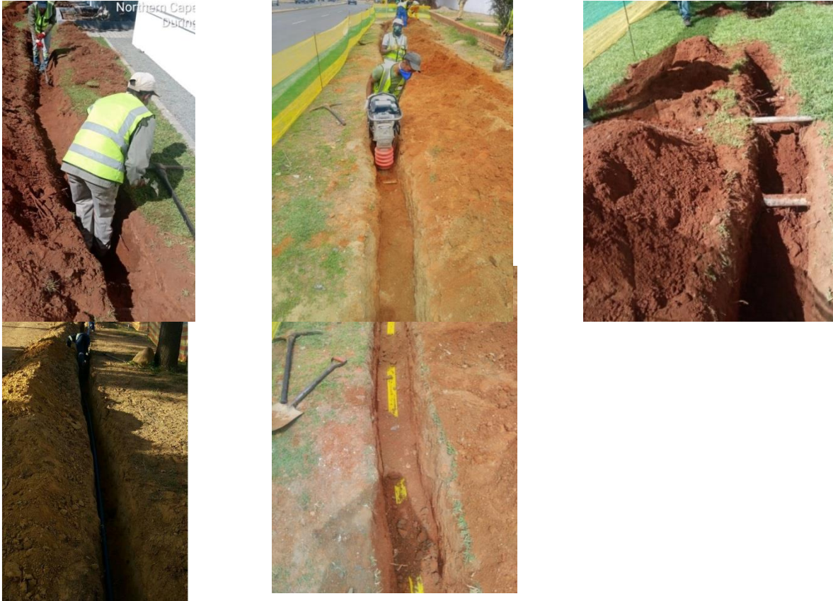
Figures 12 - 14: Some photographs of conventional trenching within the Sol Plaatje Municipal area
