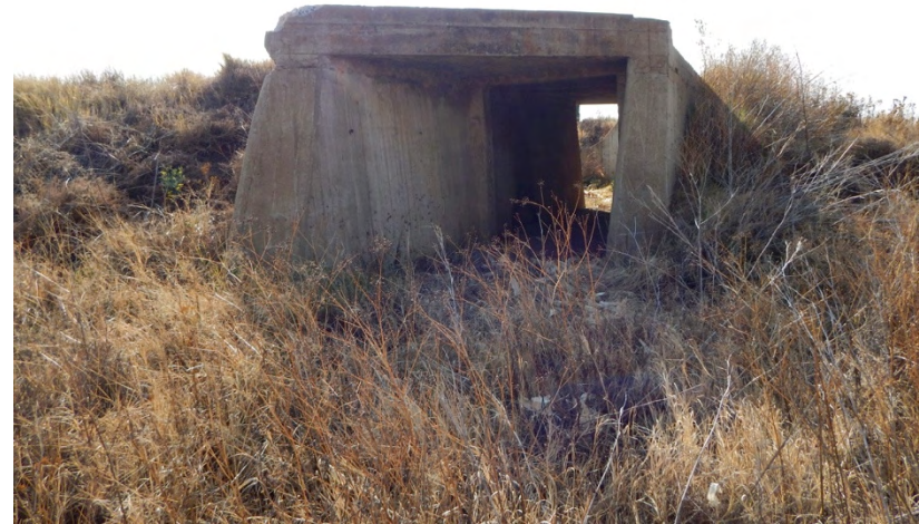
Figure 53: Entrance to the remaining structure of the explosives storage magazine (within lease area)
