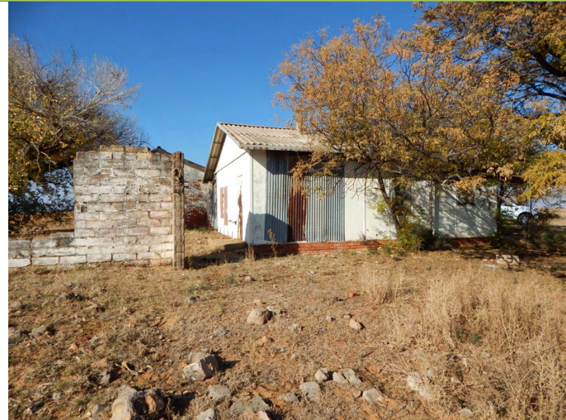
Figure 41: Dilapidated remains of a historic building (outside lease area, within mining right area)
