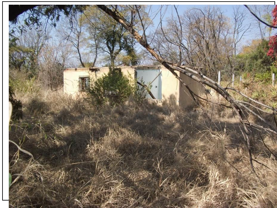
Figure 14- The August 2017 survey revealed that HH01 has fallen in total disrepair (below).
