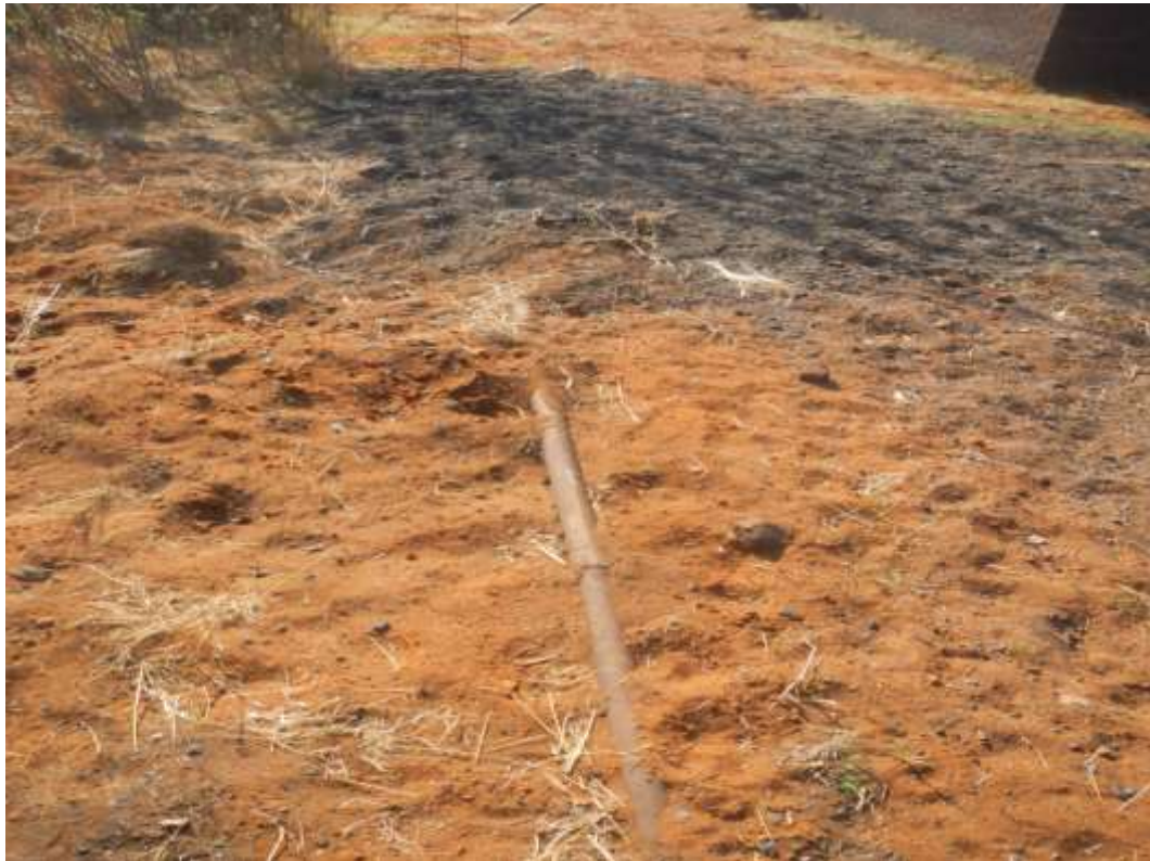
Figure 9: An exposed supply pipeline running along the railway line
