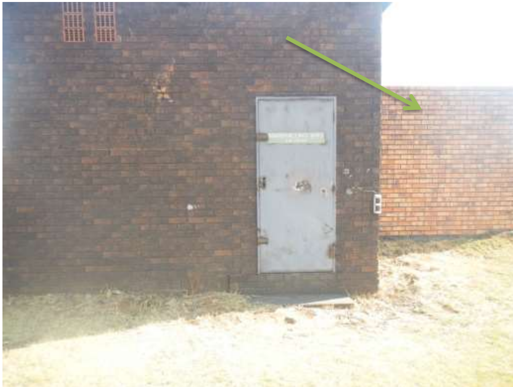
Figure 11: The Marshall Yard electricity substation
