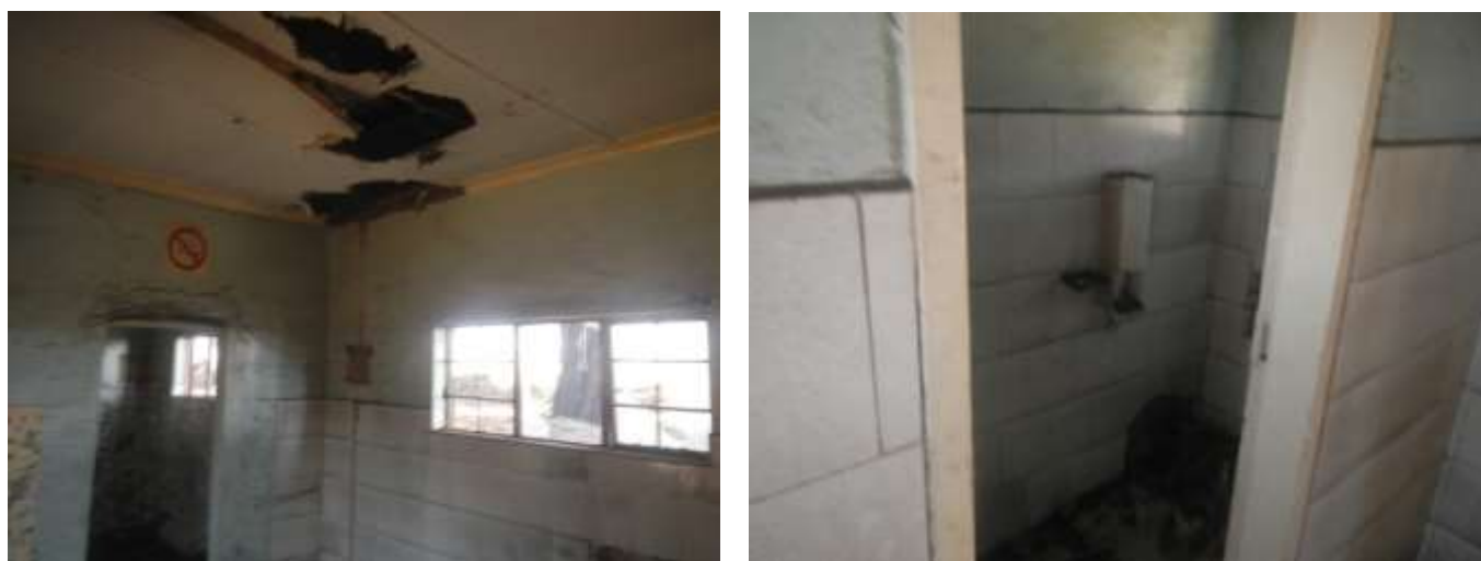
Figure 13: View of the dilapidated inside of the abandoned red-cross building
