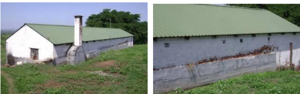
Figs 7 and 8: Showing the old brick barn: the portion towards the trees is in English bond suggesting that this portion was pre- or immediately post- World War II.
