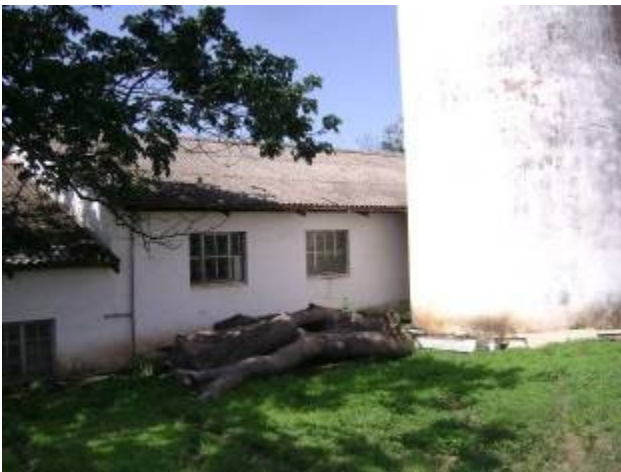
Figs 5 and 6: Showing grouping of silos, barns 1 and 2 and brick barn, and extended portion of barn no 1 with silo in foreground
