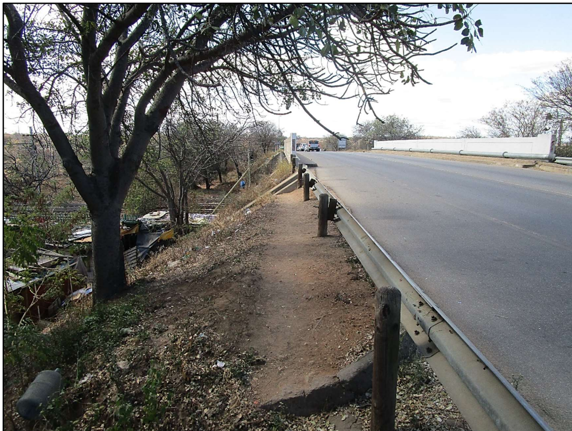
Figure 14. A view of the bridge over the railway line road D5012 - easterly direction.
