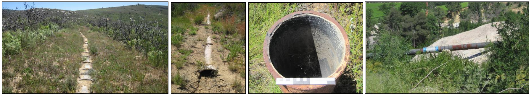
Plate 4: Partially exposed gravity feed concrete pipe sections between the Nantes and Bethel Dams. Plate 5: Exposed asbestos cement (?) pipe en route to the spring. Plate 6: A section of abandoned iron pipe at waypoint 007. Plate 7: Sections of iron pipe are elevated above granite outcrops en route to the Ysterbrug pump station.
