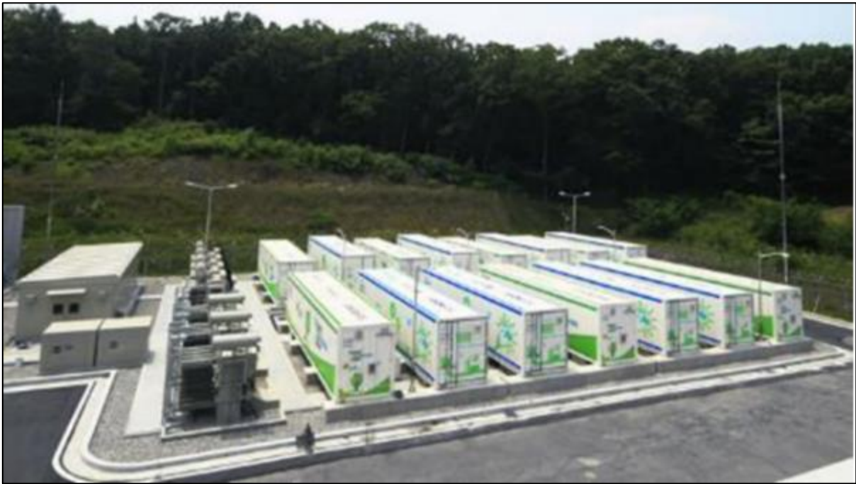
Figure 8: Example of a 15-container Lithium-Ion BESS installation.
