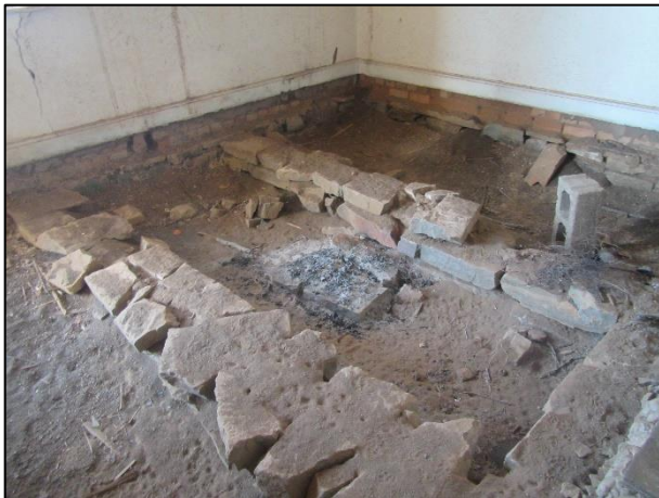
Figure 86: A vandalised floor in the main house at waypoint 1791 in HL04.
