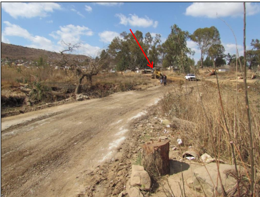
Figure 5-5: Existing Stoffel Park Project area being levelled by a grader (shown by arrow) at time of heritage screening assessment
