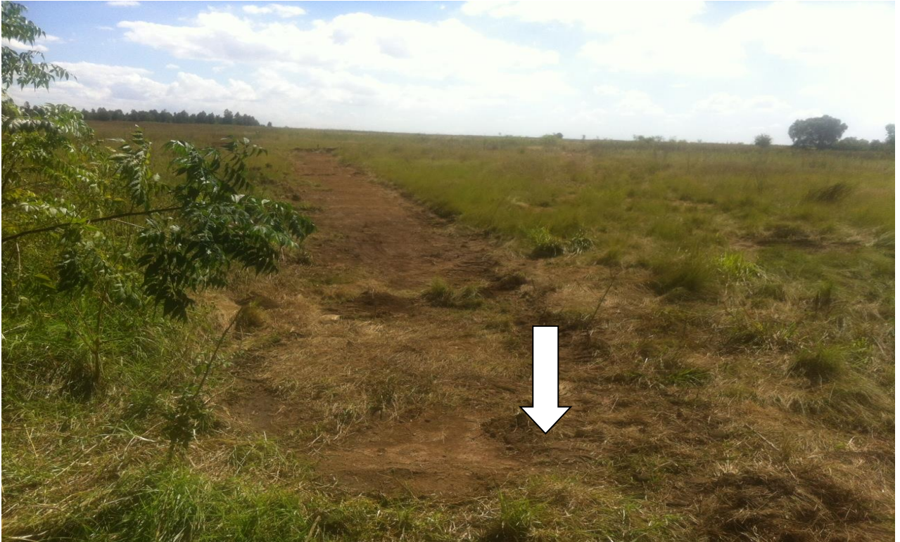
Plates 1: Shows the cleared sewer pipeline route. Note that clearance work from the marked point was halted because the pipeline route cuts through a burial site. The route will be shifted from the marked point to avoid the site
