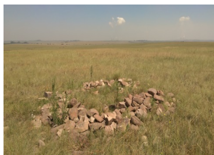
Figure 5-7: Ft-011 collapsed stone walling and foundations
