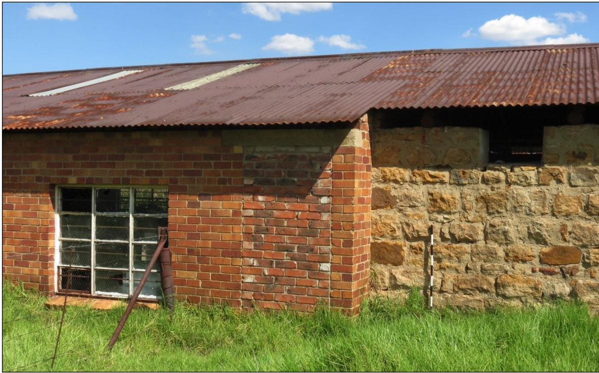
Figure 30 – Different phases in the construction and use of the building can be seen from this image. The brick sections on the left would have represented a second or potentially third building phase with the sandstone component on the right potentially younger than the sandstone section on the south-eastern end of the site.
