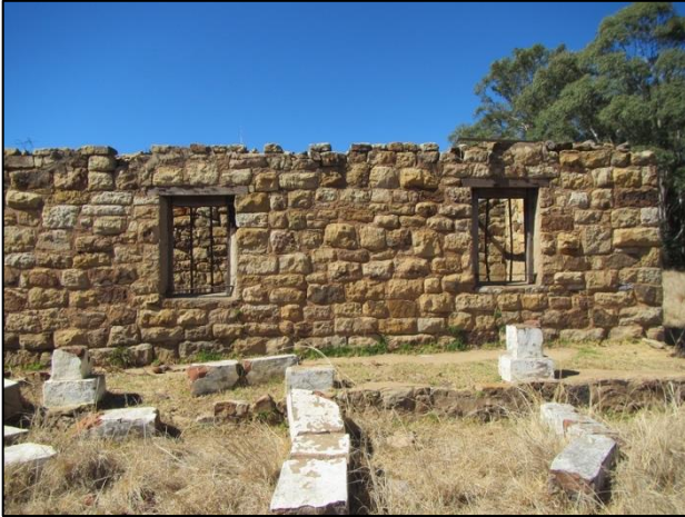
Figure 30 – Front of ILM007 showing collapsed pillars
