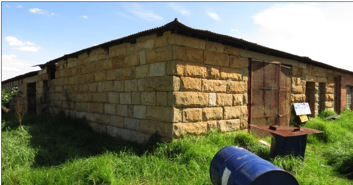
Figure 29 – The south-eastern corner of the building representing what appears to be the oldest component of the site. Sandstone lintels above the window and door openings can be seen on the right.
