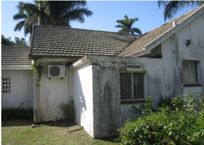
Fig 55: General view of rear of house – note issues with damp and maintenance
