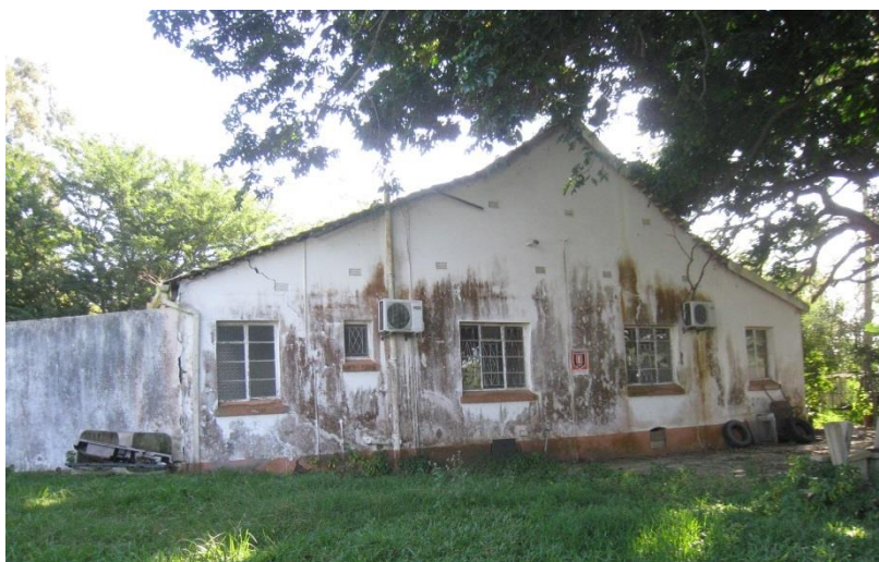
Fig 41: East elevation (under large tree). Note damage to walls
