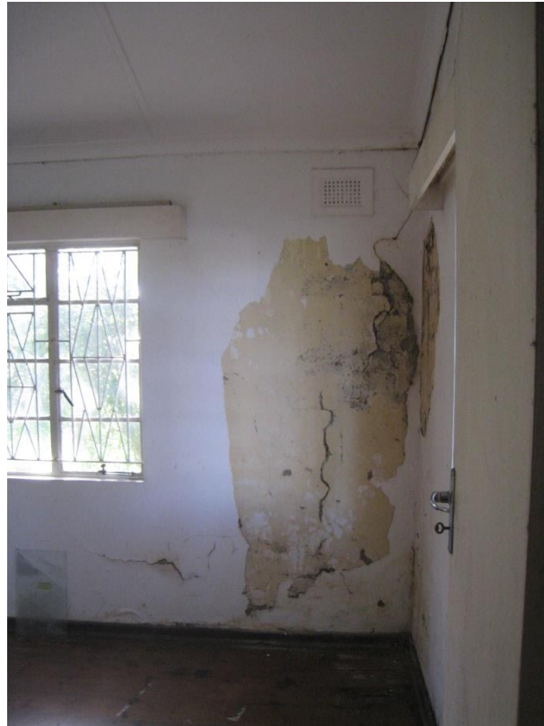
Fig 33: Structural crack in the east wall
