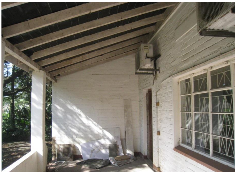
Fig 37: View along the front veranda showing collapsed veranda wall to the left
