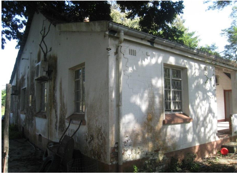
Fig 39: North east corner of House 1. Note structural cracks probably from roots
