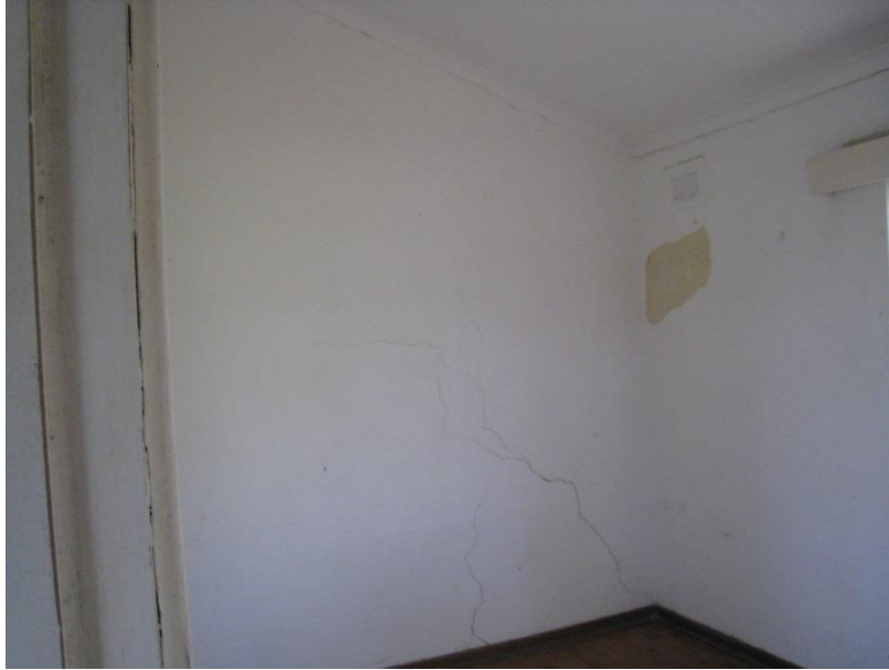
Fig 32: Showing significant structural crack (eastern side of the house)
