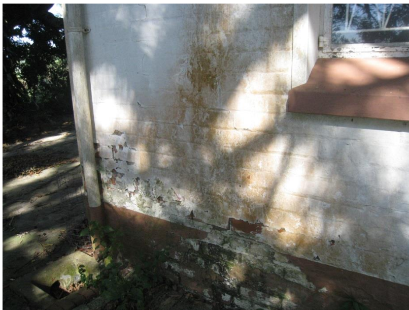
Fig 27: Drain and detail of material damage to the north east corner on the front elevation
