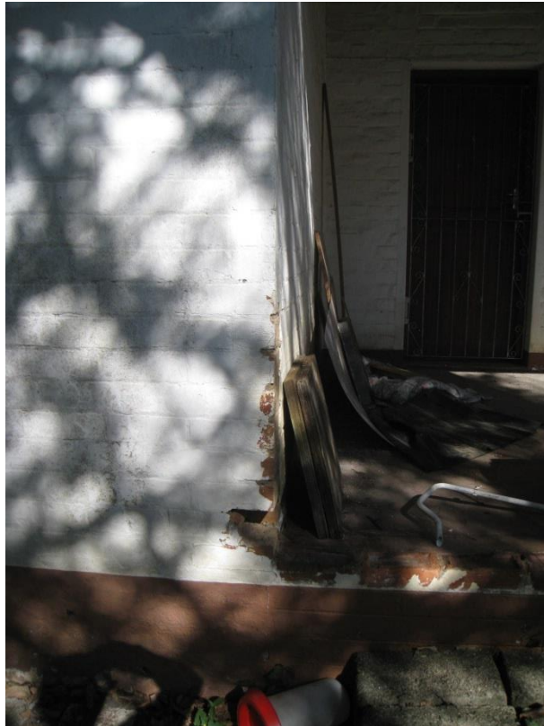
Fig 28: Damage to the stoep wall, north facing elevation
