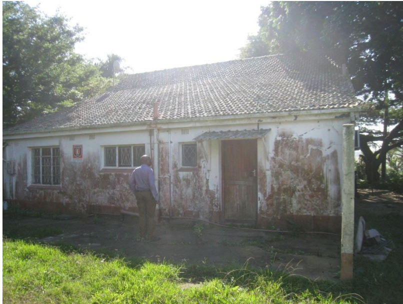
Fig 26: South entrance to House number 1 – note large trees in the proximity, possibly contributing to the structural damage to the walls
