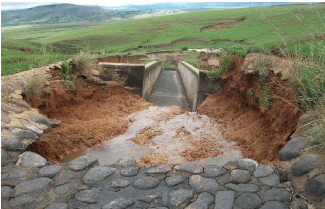
Figure 5: Canal / storm water drain with erosion and project area in background
