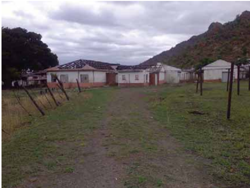
Figure 41: Some of the hospital buildings with corrugated iron roofs removed.
