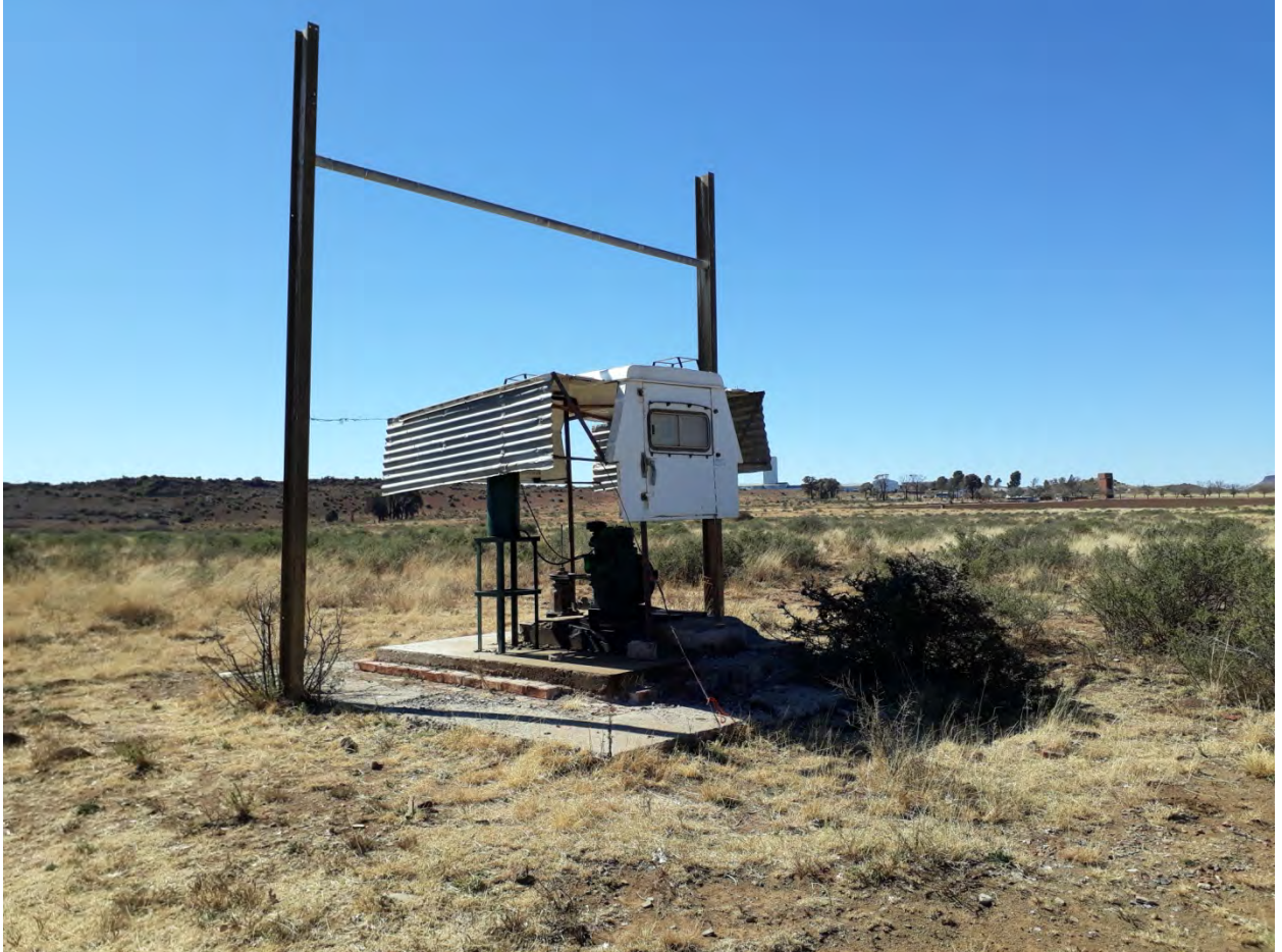
Figure 13. Modern pump station, Area 2.
