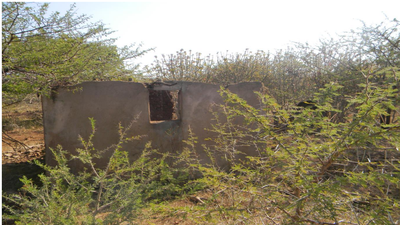
Plate 14: Photo 14: View of dilapidated structures within the mining development site (Photograph © by Author 2017)
