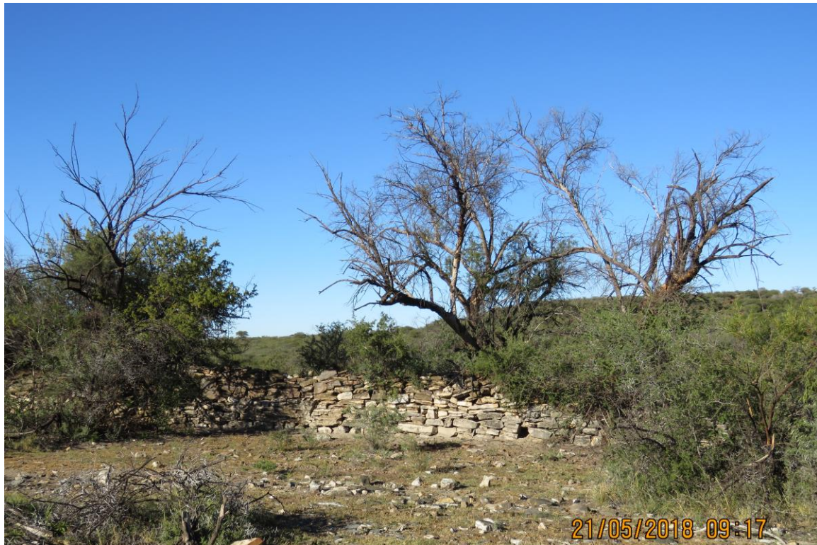
Figure 18. Portion of one of a few (partially washed away) dam walls across the valley. Observation 9.
