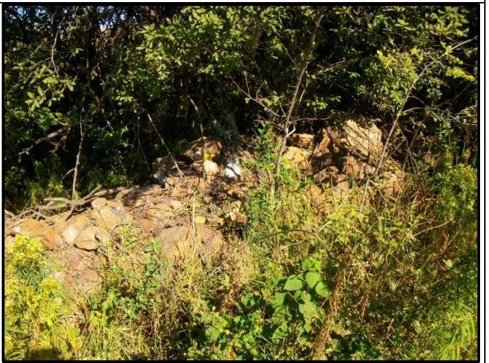
Figure 24: Overgrown Stone walling at Site 5
