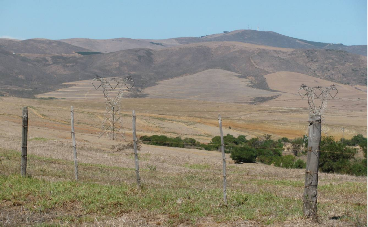
Figure 8 4x400 kV transmission lines close to Kalkfontein (above) are quite well absorbed by the rolling landscape despite the fact they are only 340 m from the visual reference point.
