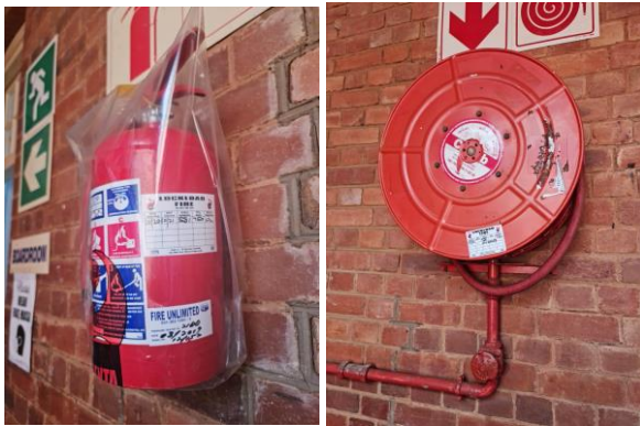
Figure 12: Fire Extinguishers and Signage installed
