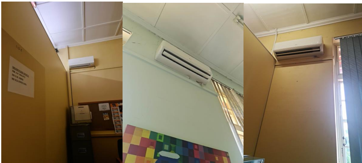
Figure 9: Room 115 (115a, 115b and 115c) aircons
