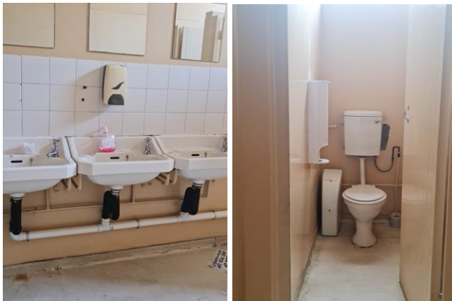
Figure 15: Drainage pipe need to be maintained (Room 35)
