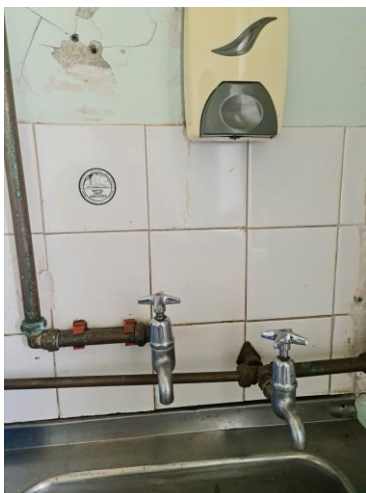
Figure 13: Hot & Cold-Water pipes need to be replaced
