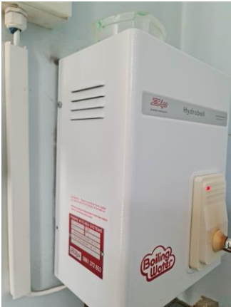
Figure 21: Ground floor admin hydro boil need replacement
