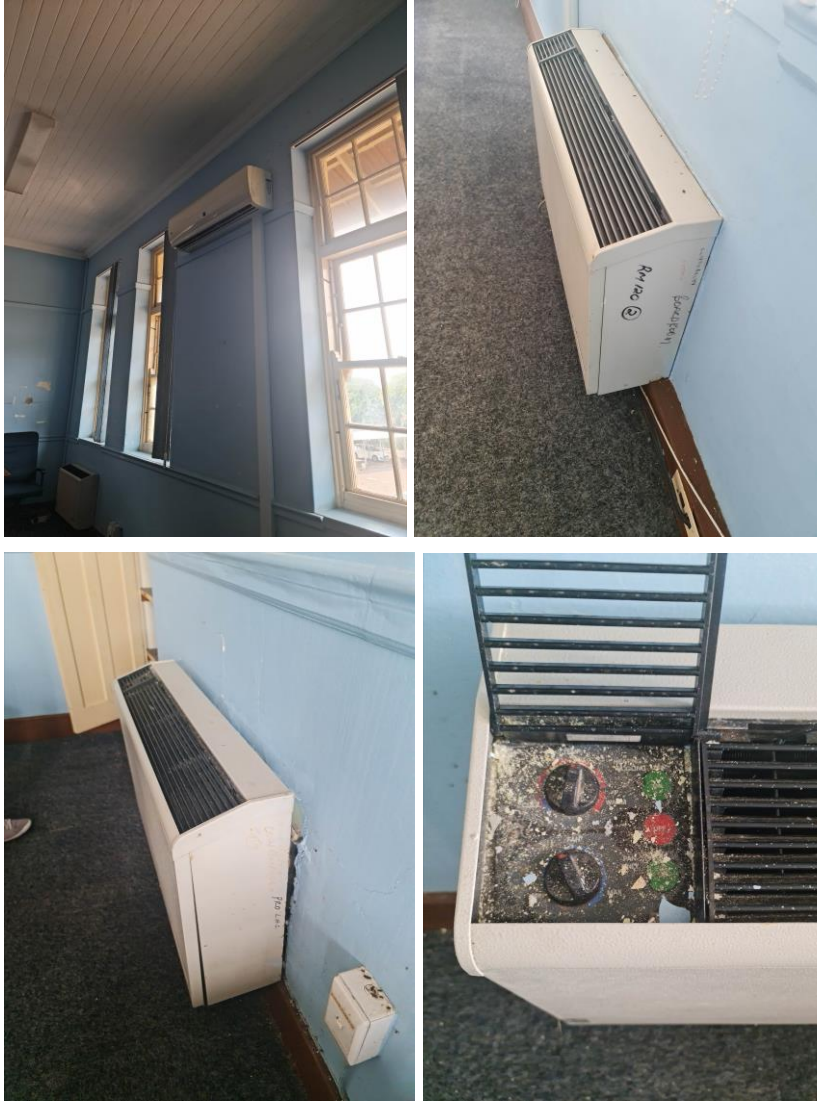
Figure 2: First Floor Boardroom aircon
