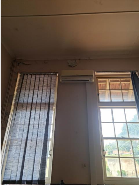
Figure 6: Room xx aircon is old and need to be replaced
