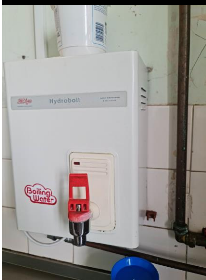
Figure 17: Hydro boil need to be replaced
