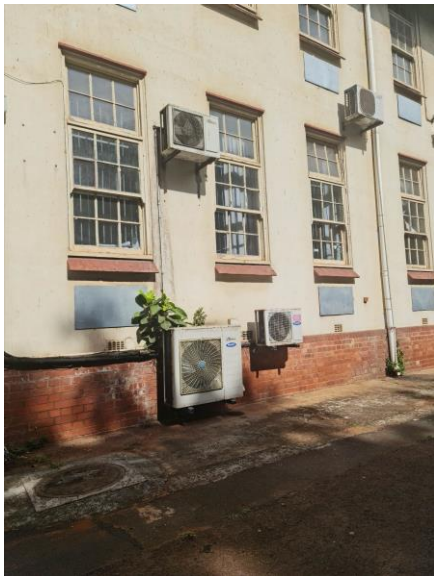
Figure 1: MLB Building Outdoor Units
