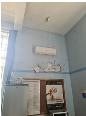
Figure 10: Ground floor Admin office Room 26 aircon
