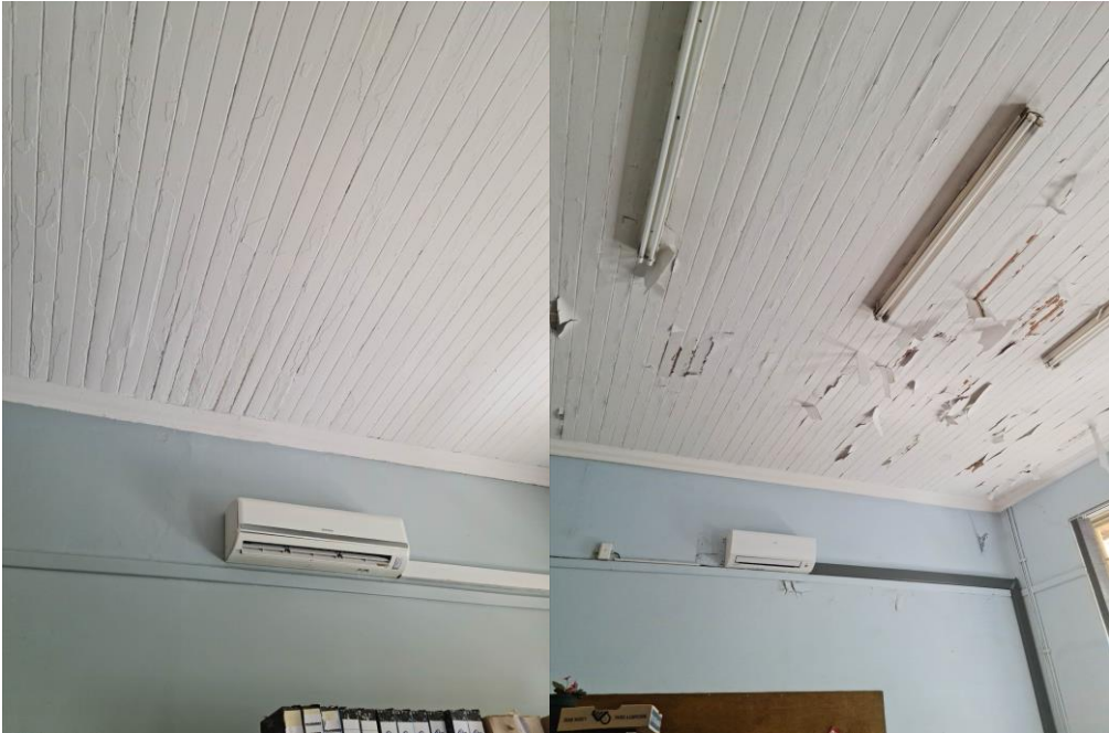
Figure 7: Rooms 116 & 118 aircons are old
