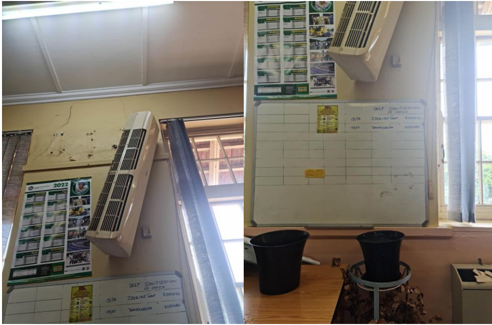
Figure 8: Room 114 aircon is broken and not working
