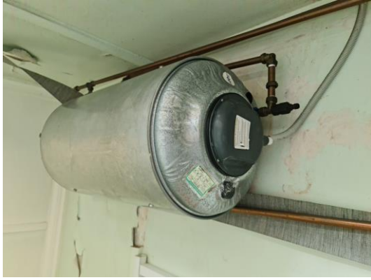
Figure 14: Geysers 100L need maintenance
