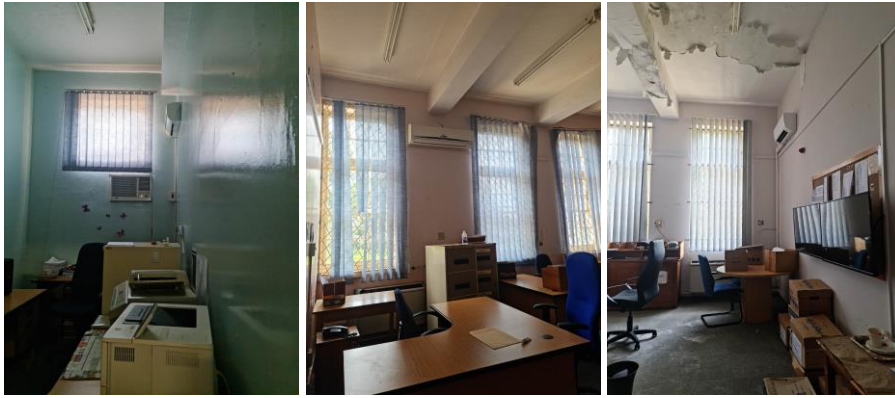
Figure 11:Ground floor Rooms 30, 30a and 33a aircons
