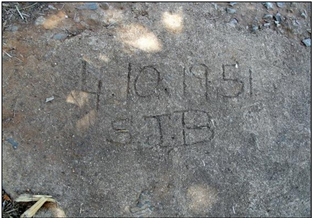
Fig. 28. Site KP 23. This date inscribed on the concrete of the canal and weir structure suggests that the structure is 64 years old.
