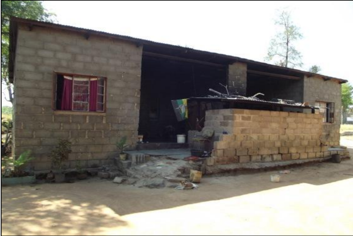
Fig. 9. Site KP 8. Farm worker's house, split unit. Photo taken in eastern direction.
