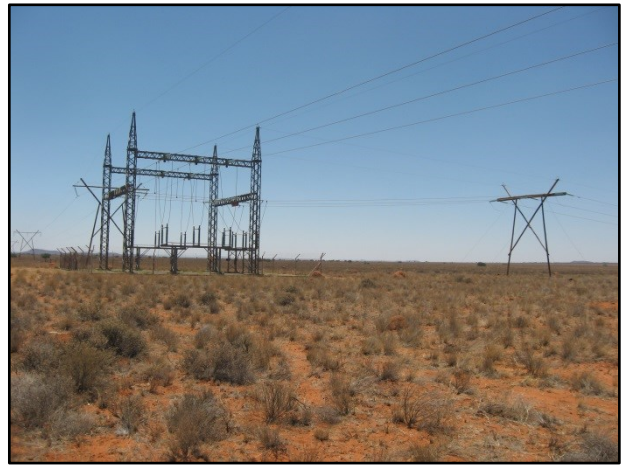
Figure 5 – View of the substation and the power lines
