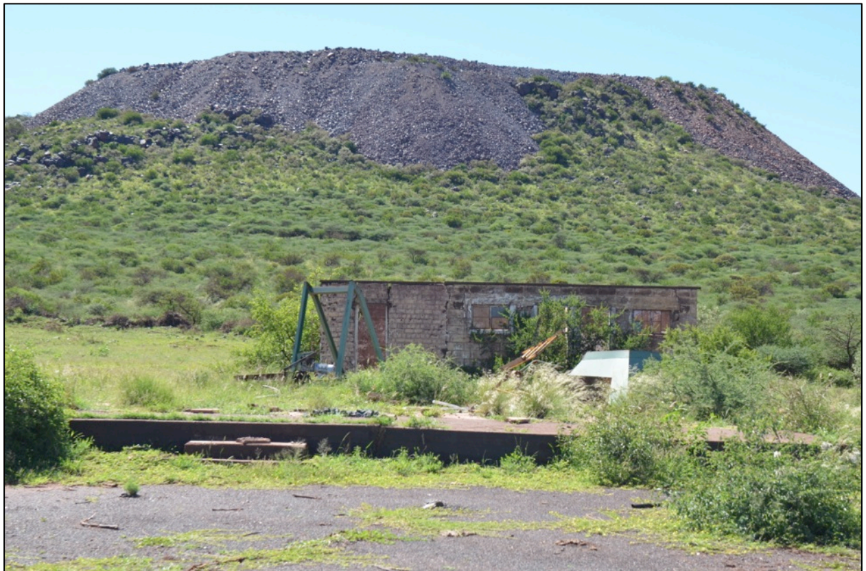
Figure 34. Dilapidated building at Site 7
