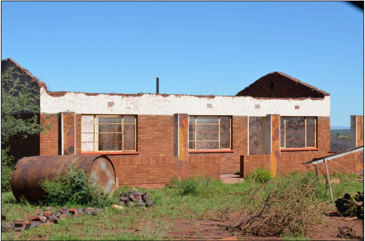
Figure 35. Dilapidated housing structure at Site 7
