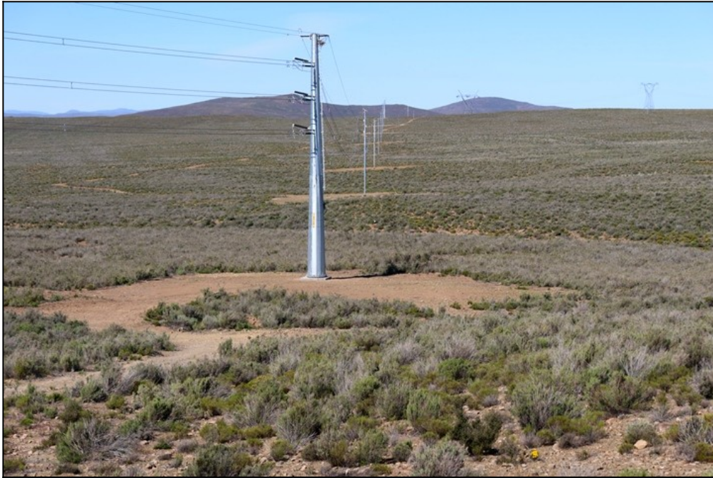
Figure 10: View eastwards along the recently constructed powerline between the new substation on Bon Espirance 73 and the Komsberg MTS. Bedrock exposure in the low relief terrain here is very limited. Any palaeontological impacts are more likely to be attributable to surface clearance than to excavations for electrical pylon footings.
