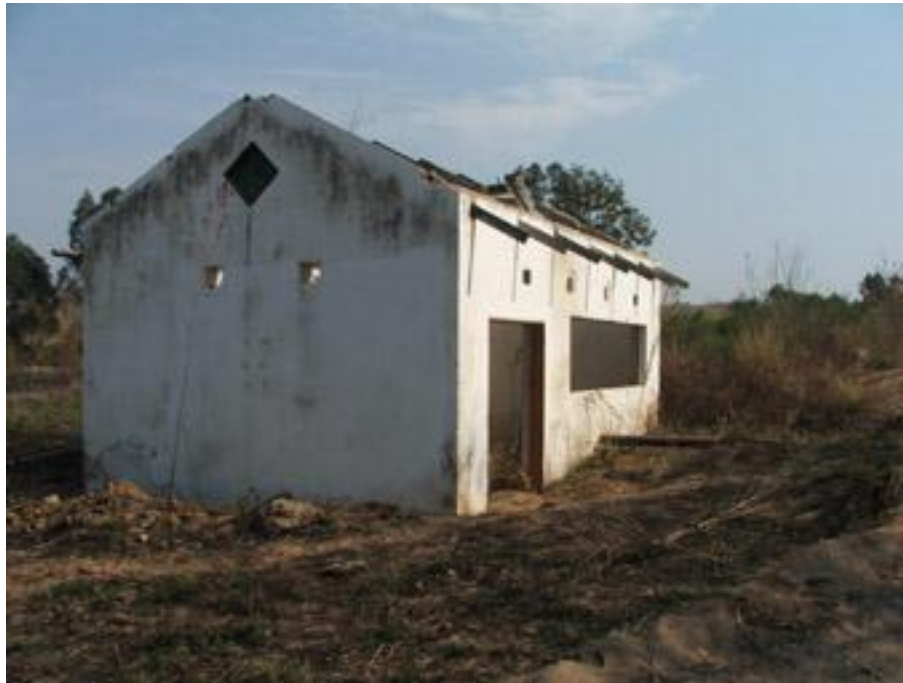
Figure 24. A pump room located at Site 18.
