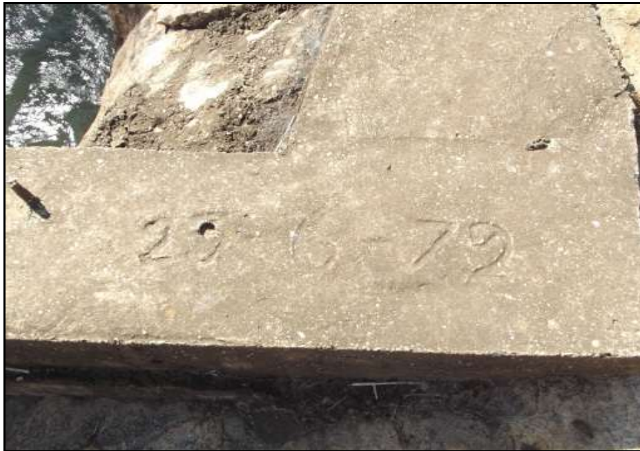
Fig. 8. An date at the sluice gate probably indicates when the current sluice gate was installed, 23 June 1979.
