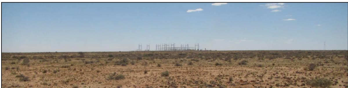
Figure 3: View towards the northeast (from the PV 1 site just north of the railway line) of the Nieuwehoop Substation currently under construction.
