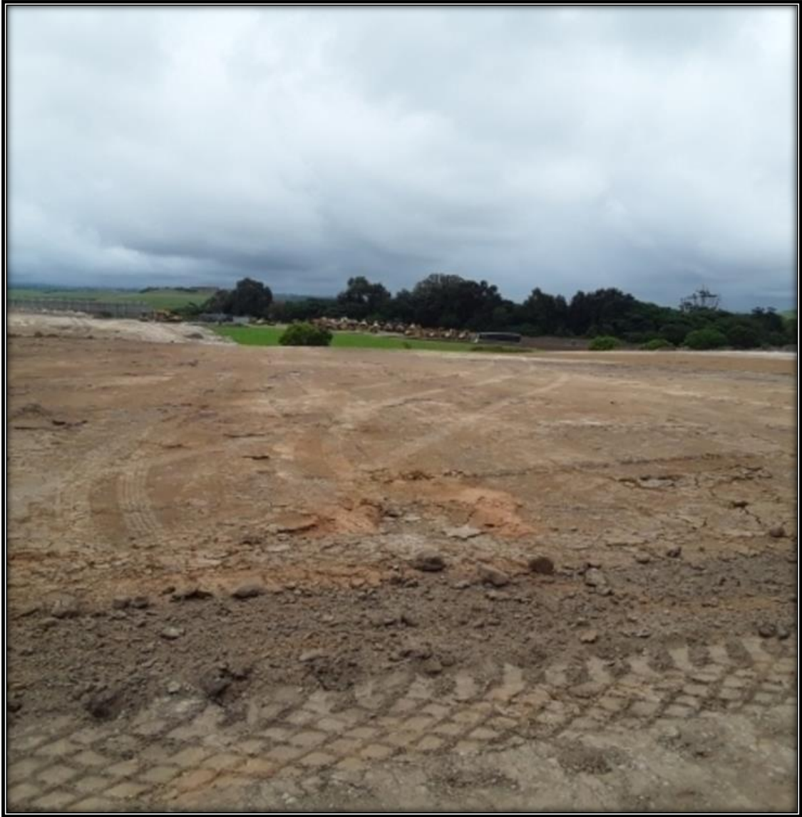
Figure 10:Vegetation clearance exposing the surface of the proposed development GPS coordinates - - 29.615000S; 31.098056E
