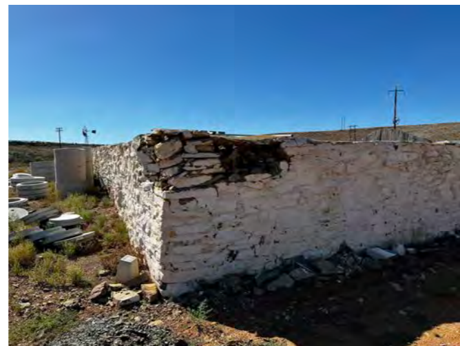
Figure 51: Damaged portion of kraal wall
