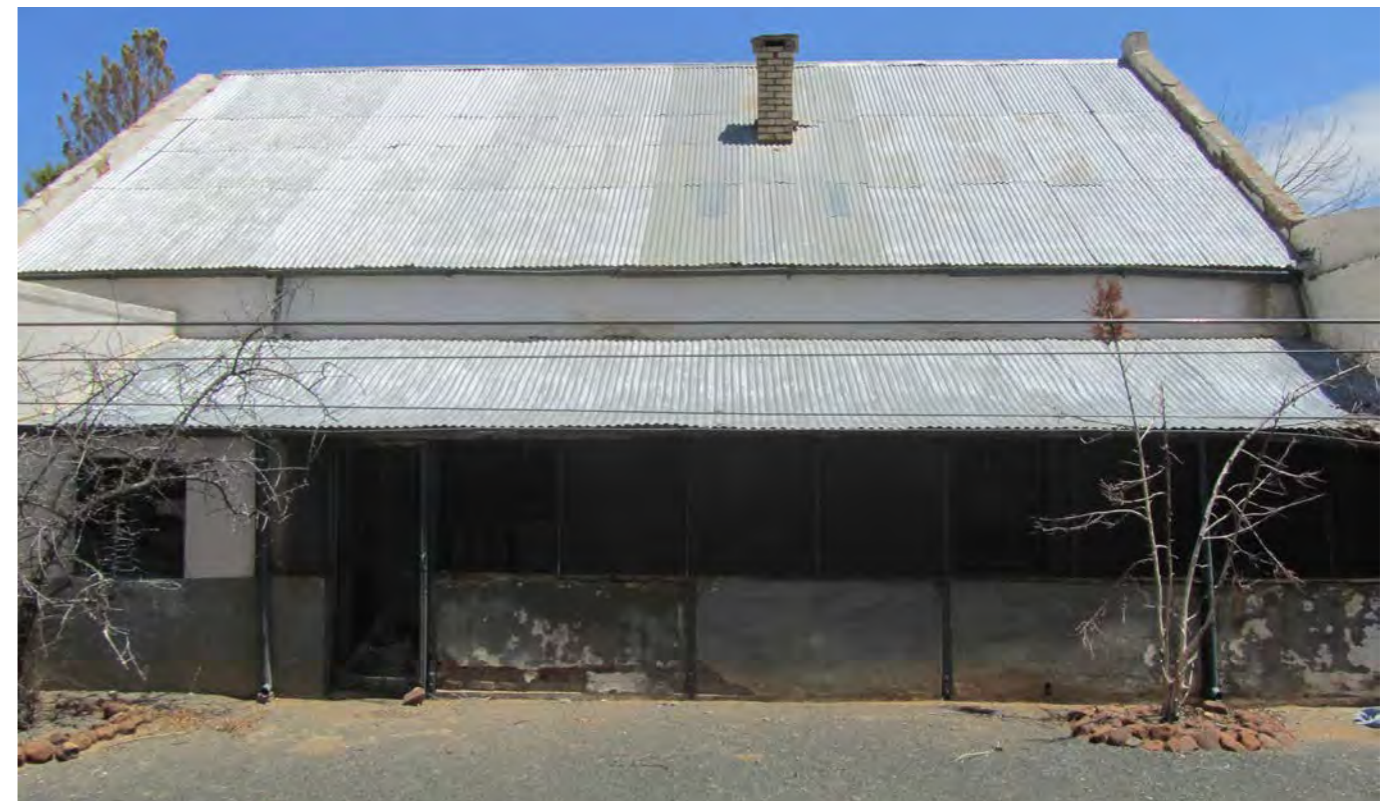
Figure 26 & 27: The front stoep of the Klerefontein farmhouse in comparison with the Front stoep at the Groot Paardekloof farmhouse. The original Klerefontein stoep design was likely similar to that of Groot Paardekloof.
