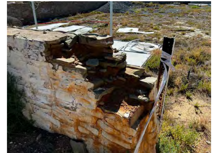
Figure 55: Damaged portion of wall
