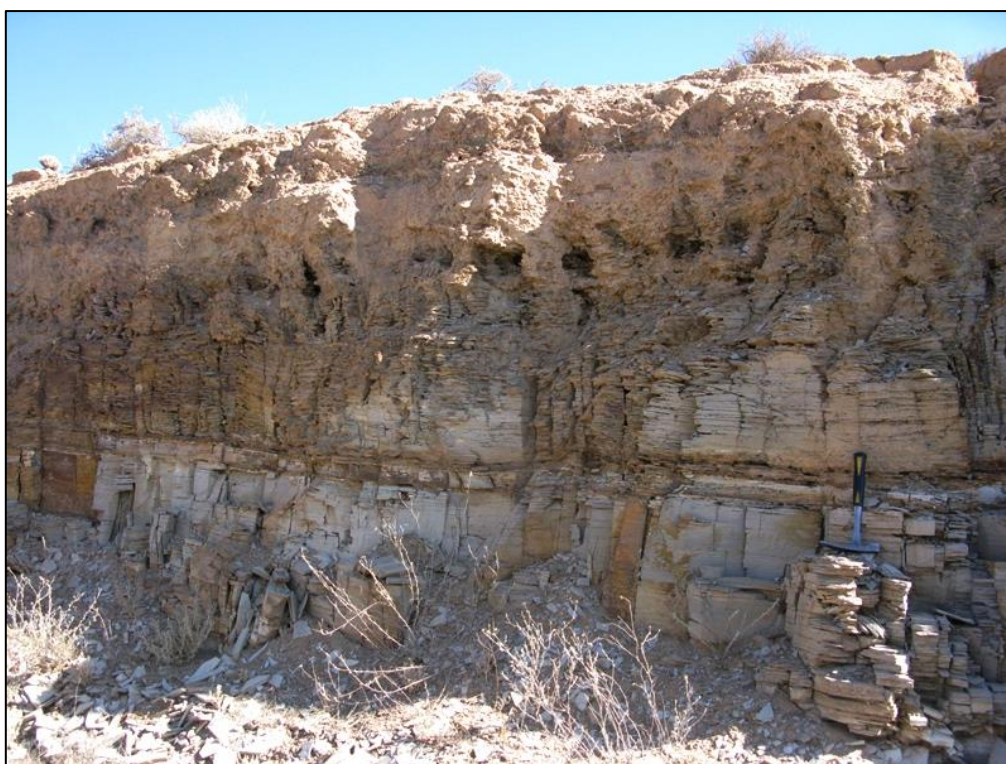
Figure 14: Borrow pit cut face section through gently-dipping, tabular-bedded mudrocks of the Whitehill Formation overlain by saprolite and thick, silty, gypsiferous soils (Loc. 261) (Hammer = 30 cm).
