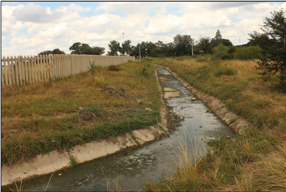
Figure 3: Concrete storm water drainage system outside the development footprint
