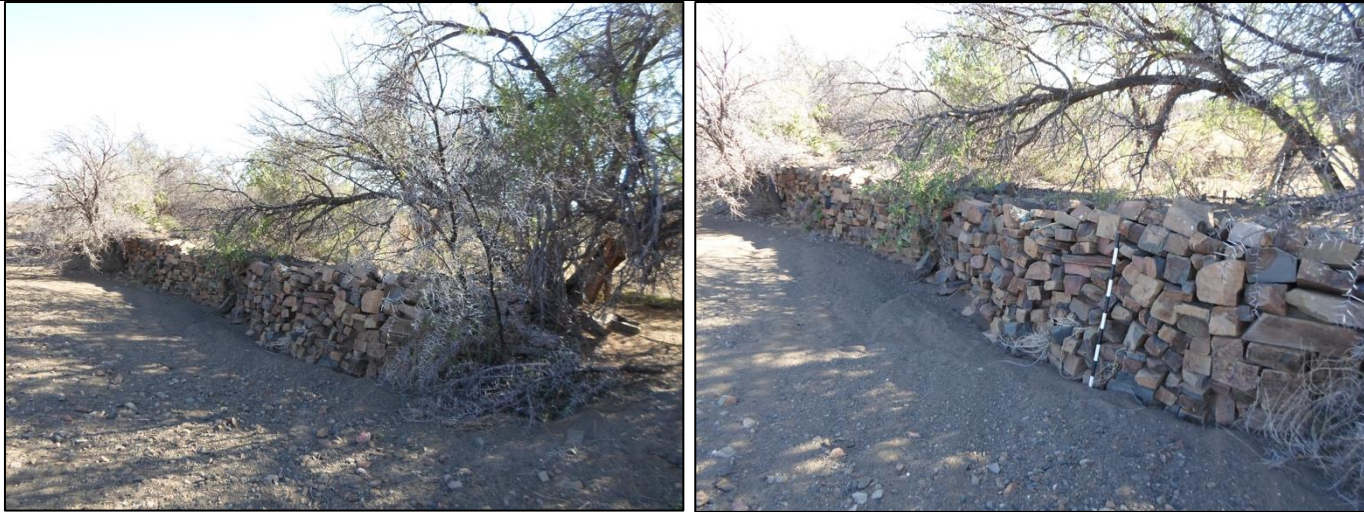
Figure 31: View of the packed stone wall or water break in the nearby stream at K012/4.
