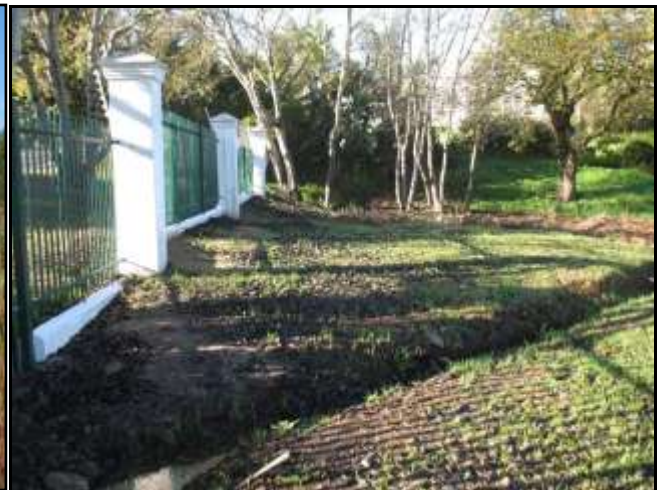
Figure 6: Gabions will be built around these pipe outlets at the far east end of the study area.
