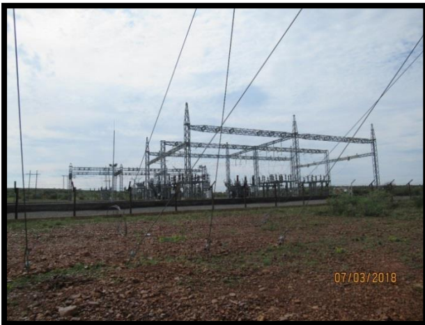
Eldoret SS – expansion will be on the area in the foreground. Work has not started here.
