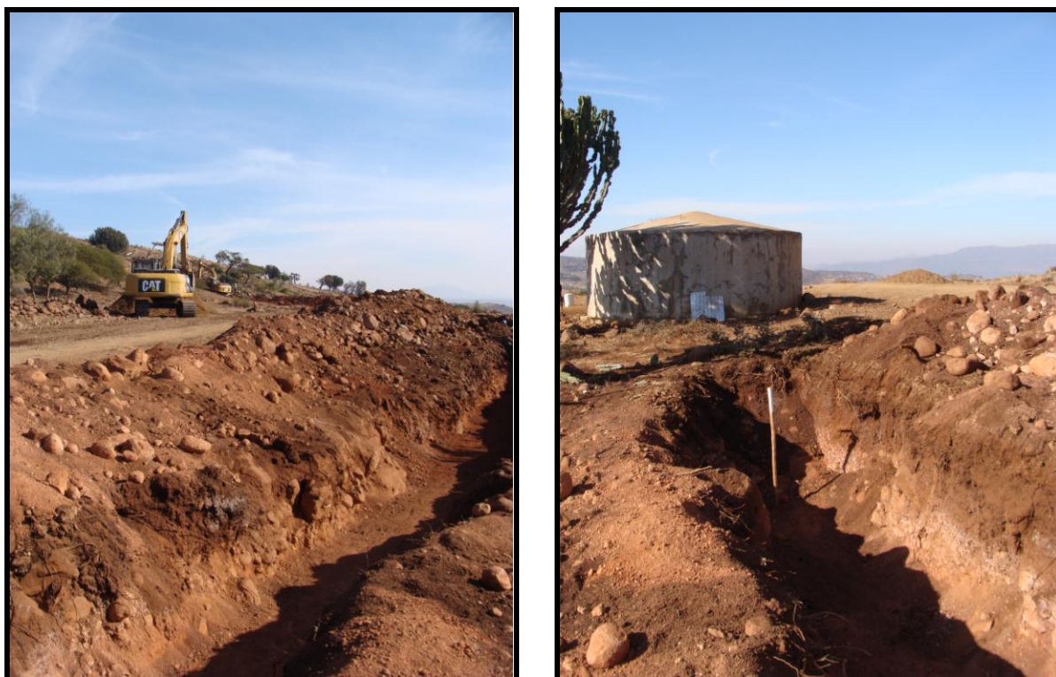
Figure 14 & 15: On top of a dolerite hill a construction crew were busy digging the trench leading up to one of the existing reservoirs, which will be replaced with a new 350kL concrete/steel reservoir. Another team of workers was inside the completed section of the trench and were preparing the base of it for the laying of the pipe. The specifications given for the trench is that it is to be 0.8 m wide, but this ditch considerably exceeded that. The reason for this could be because of the fact that this bedrock was non-fossiliferous and caution wasn't needed to be exercised, or because it was maybe a more difficult rock-type to excavate
