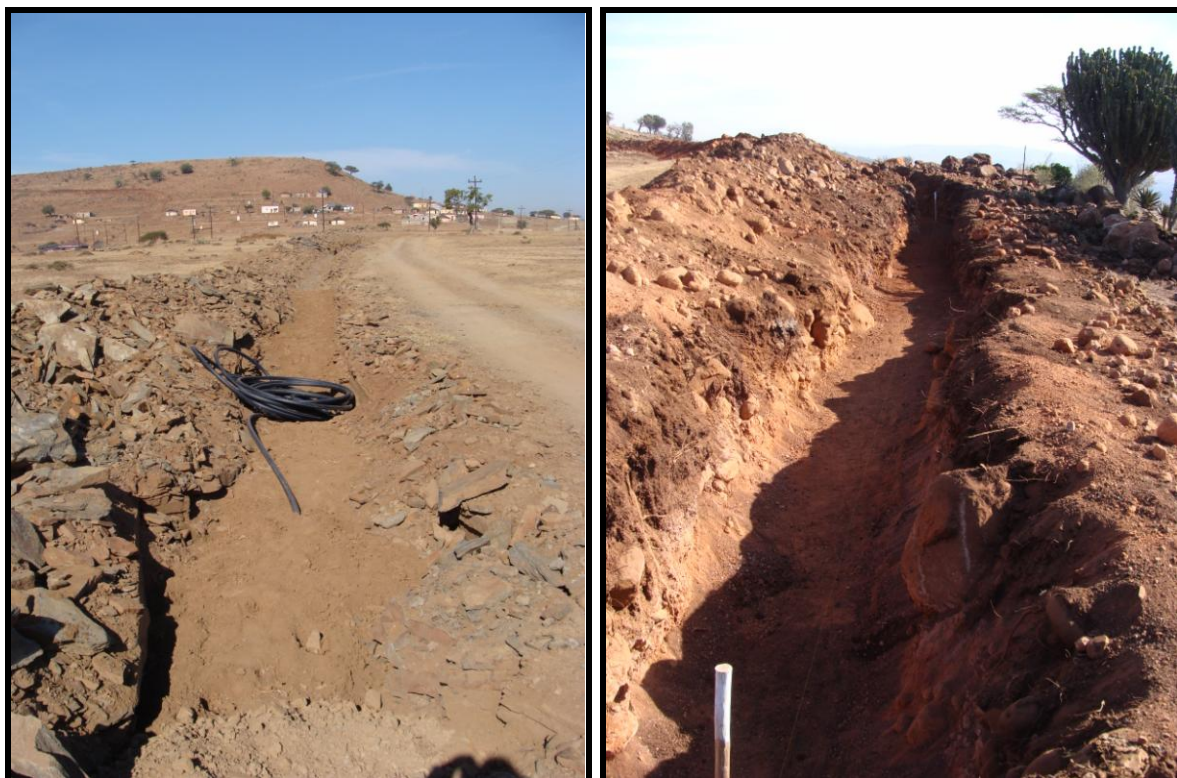
Figure 12 & 13: Sections of the pipeline network had already been laid (left), and new trenches were actively being dug and prepared (right). In Fig.12 the bedrock is fossiliferous shale and immediately to the right of this photo is the quarry where the fossils were recorded. In Fig.13 the bedrock is dolerite
