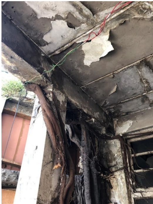
Figure 11: An internal view showing decay of steel in overhead slabs and a tree growing into the building, May 2021. Source: Chantal Pieterse
