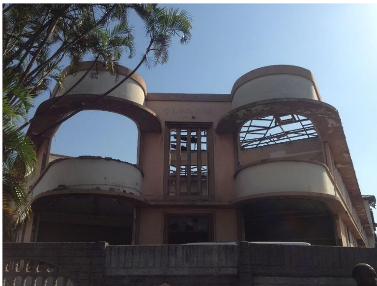
Figure 18: The building had been stripped when first visited in 2015.
