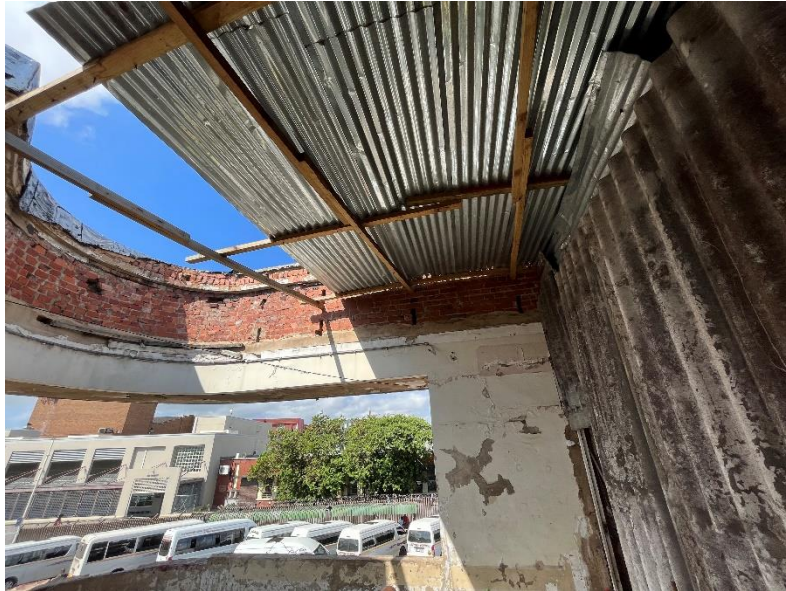
Figure 15: A makeshift roof has been installed on the upper floor with a temporary wall division, May 2021. Source: Chantal Pieterse
