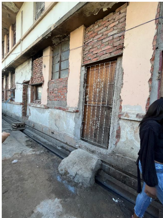
Figure 13: Infill brickwork and openings in the University Ave facade, May 2021. Source: Chantal Pieterse
