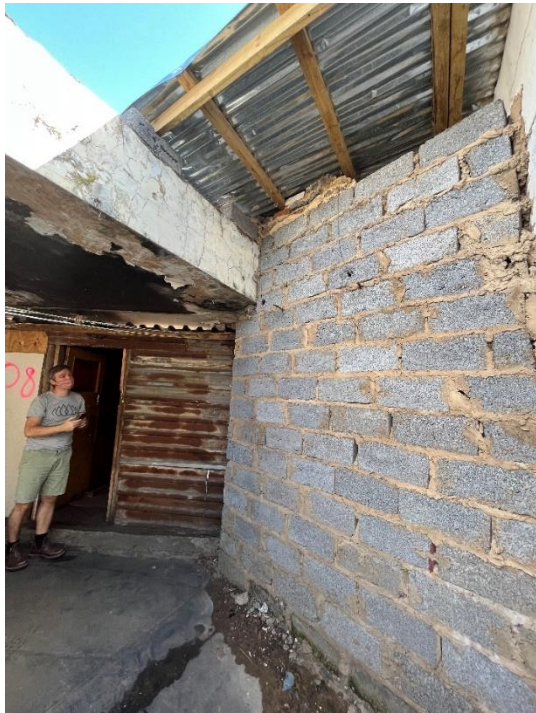
Figure 16: A makeshift roof and concrete block wall has been installed on the upper floor with a temporary wall division, May 2021. Source: Chantal Pieterse
