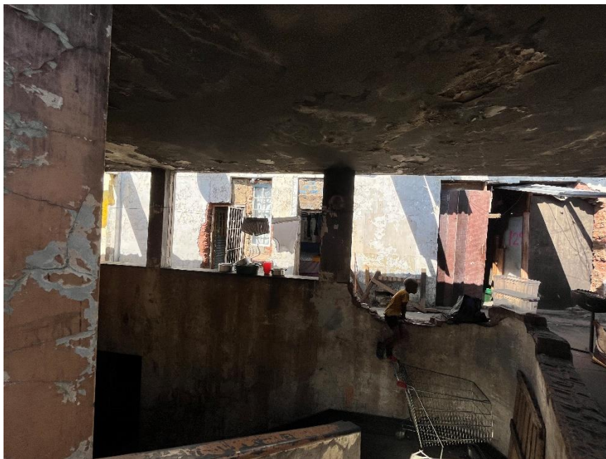
Figure 17: The internal stairs have been damaged and the upper floor is occupied, May 2021. Source: Chantal Pieterse
