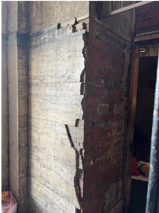
Figure 14: Marble on the entrance wall has been stripped off, May 2021. Source: Chantal Pieterse
