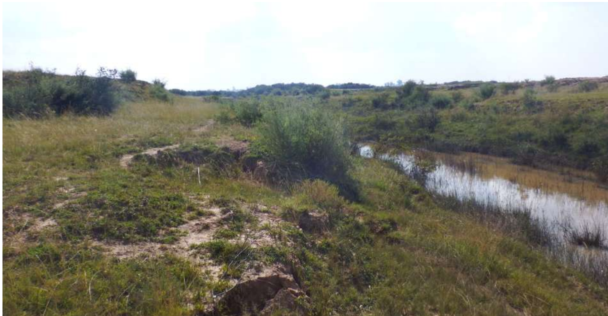
Figure 10b. The section of the pipeline for the Alternative Supernatant Discharge Point going west towards the Sandspruit are capped by superficially disturbed alluvial sediments and residual soils.
