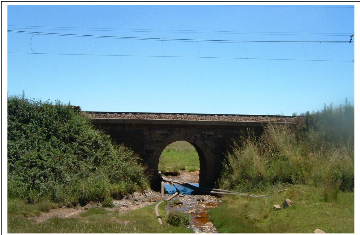
Figure 12- A bridge constructed with sandstone (HS01) carries a railway line in the Project Area. This structure probably dates from the early 20 th century (above).
