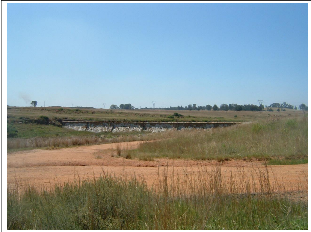
Figure 13- The Middel Dam's wall was constructed with sandstone and probably dates from the early 20 th century (above).
