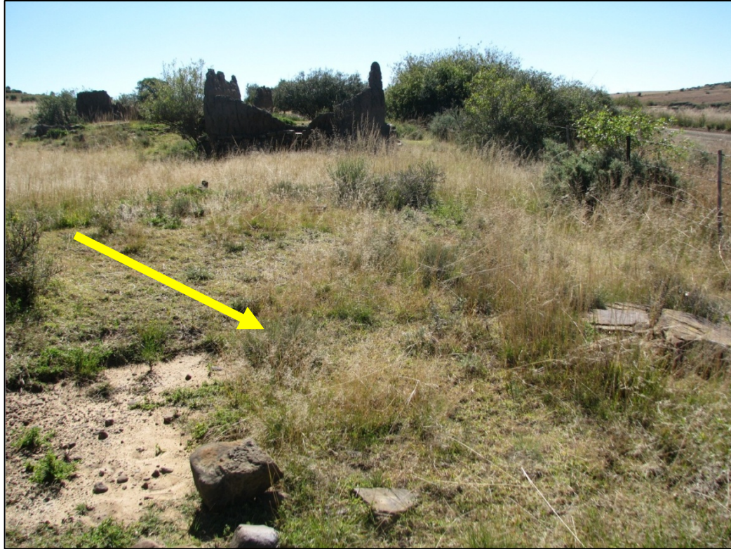
Fig. 24: The foundation of House 2 (H2) in the foreground with House 1 in the background.
