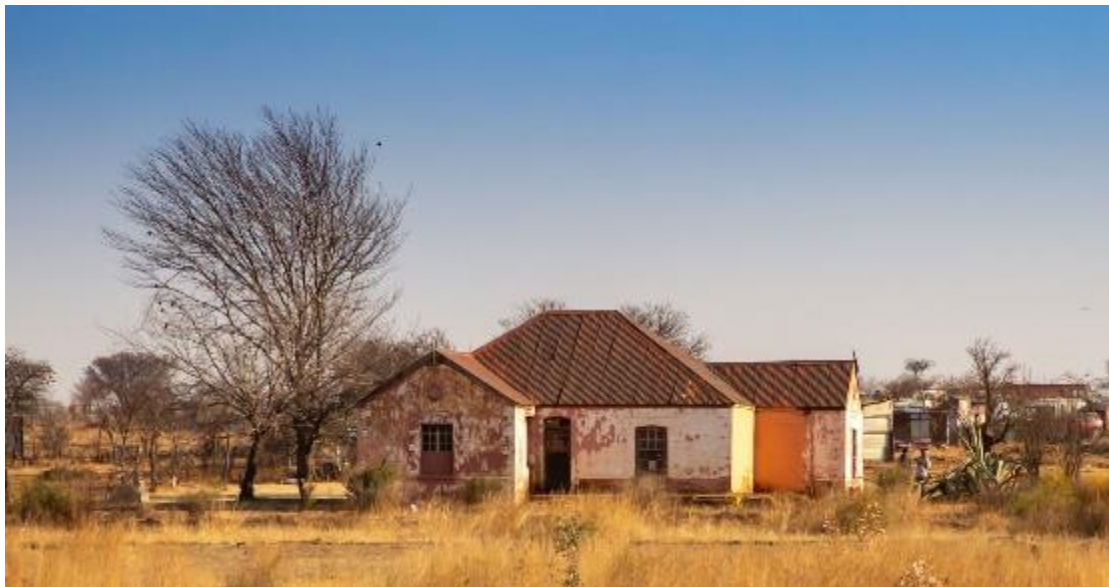
Fig. 43. Eastern elevation of the old Kwaggafontein farmhouse. Effort ought to be made to retain this structure. It is structurally sound and with a small investment it can be turned into a useful building on the new proposed schoolyard. (Photo Ziegwald Kūsel 2020)
