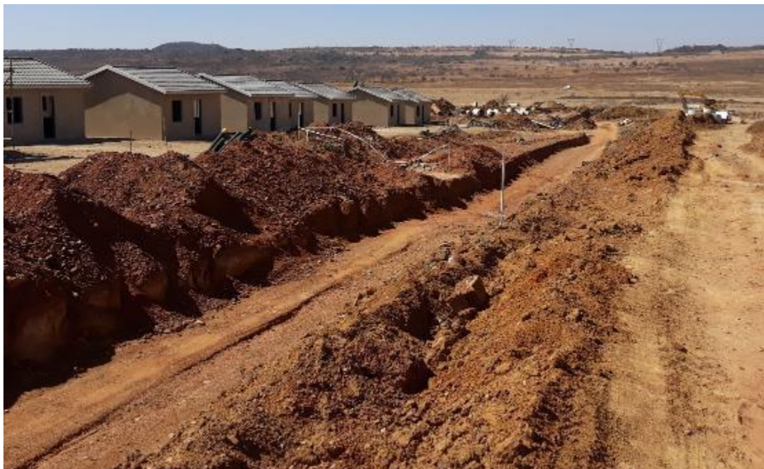
Fig. 74. Photo 65. Looking east from marker 12. New dwellings and services under construction. (Photo S.M. Miller 2020.)
