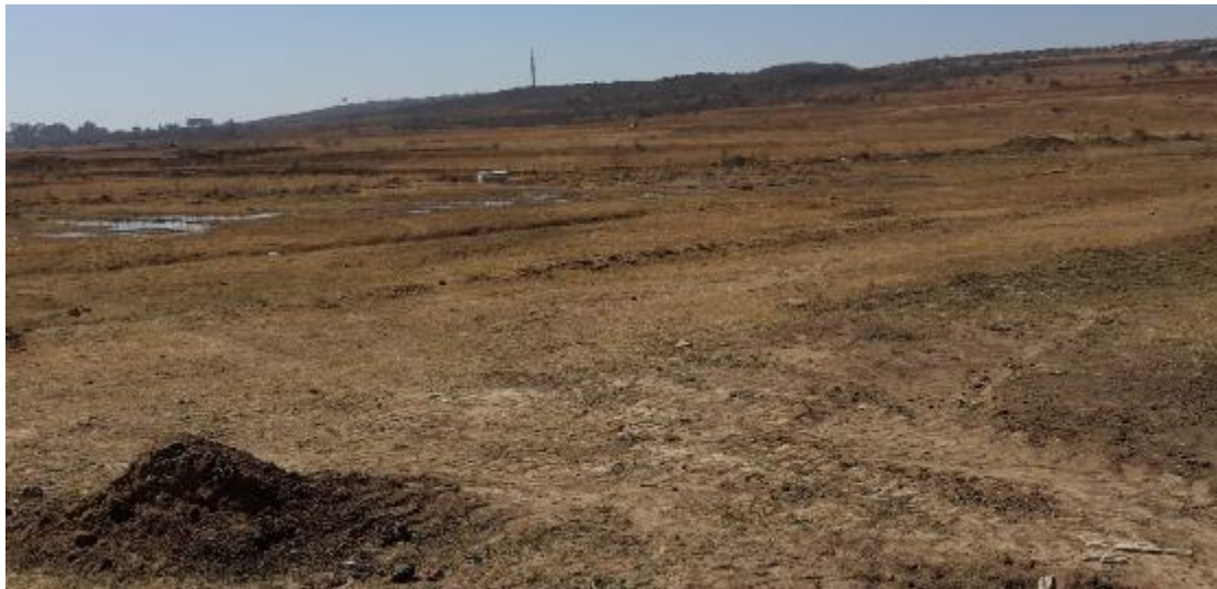
Fig. 78. Photo 65. Looking northwest from marker 14. New work in progress for roads and storm water. (Photo S.M. Miller 2020.)
